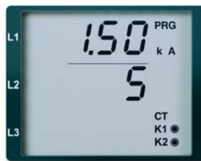
Programming of current transformer
